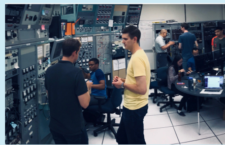
Tandem Control Room at TUNL [S71]
